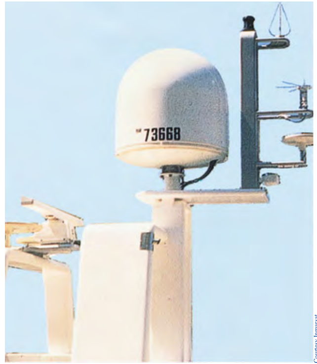
Figure 57.1 Satellite antenna ship earth station
